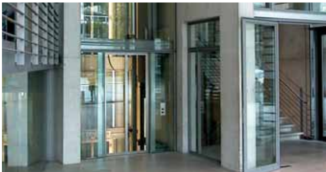
Lift fixings, guide rails
