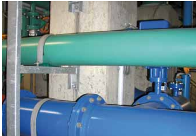
Pipe supports on vertical HZA Channels
