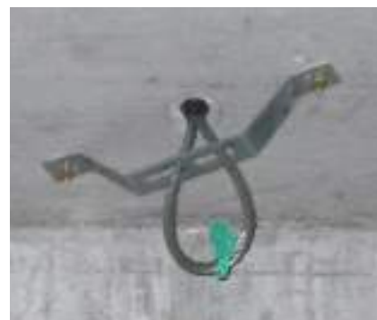
Cable loop installed in a lift shaft
